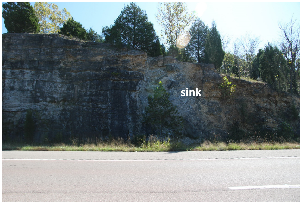
Figure 1-2. A filled sink along Highway 54 (Facing East).
